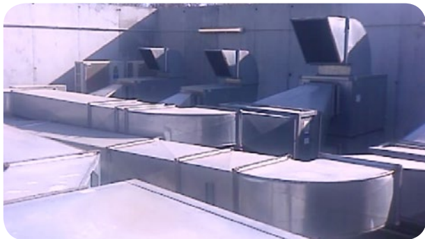
EXAMPLE OF HVAC INSTALLATION
