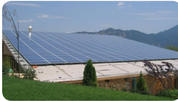
EXAMPLE OF PV ROOFTOP INSTALLATION
