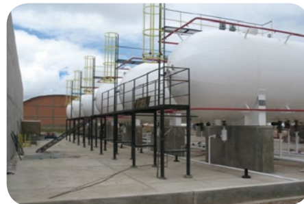
LPG STORAGE PLANT, EL ALTO, BOLIVIA
